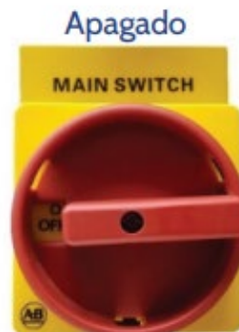
Figura 8 Swich principal en posicion off.
